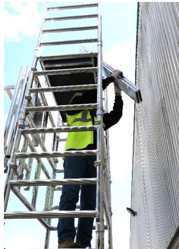
28. Relocate the toeboard assembly from the lower platform to the higher level, ensuring that it is positioned on the plain section of the platform as shown.
