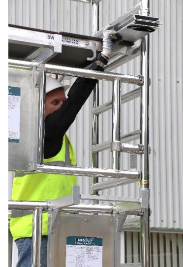
29. Relocate the toeboard assembly from the lower platform to the higher level, ensuring that it is positioned on the plain section of the platform as shown.
