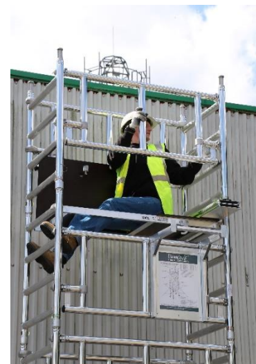
29. Fit 2 guardrail frames, with the top hook (facing outwards) set above the top rung of the frame.
