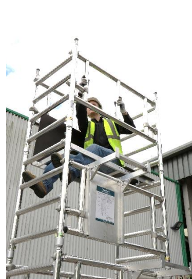
28. Fit 2 guardrail frames, with the top hook (facing outwards) set above the top rung of the frame.
